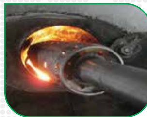
Gas Burner in Operation
