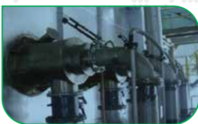
Gas Burner Mounted to a Boiler
